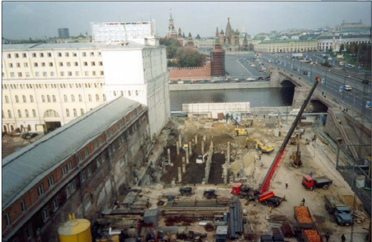
Fig. 3. Building 3. Excavation of the first layer viewed from the roof of Building 1.
